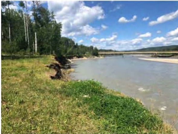
a) View looking downstream at eroding bank between bridge and pipeline right-of-way.
