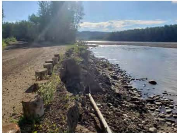
e) View looking upstream at eroding threatening access road for boat launch.
